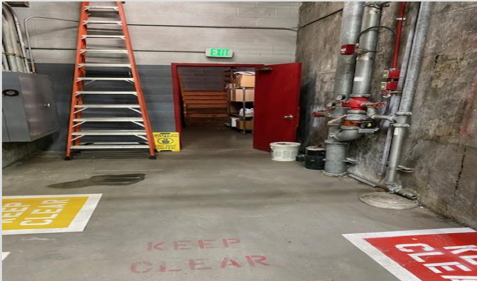
Fire exits must remain clear of obstructions and fire doors must be kept closed at all times.
